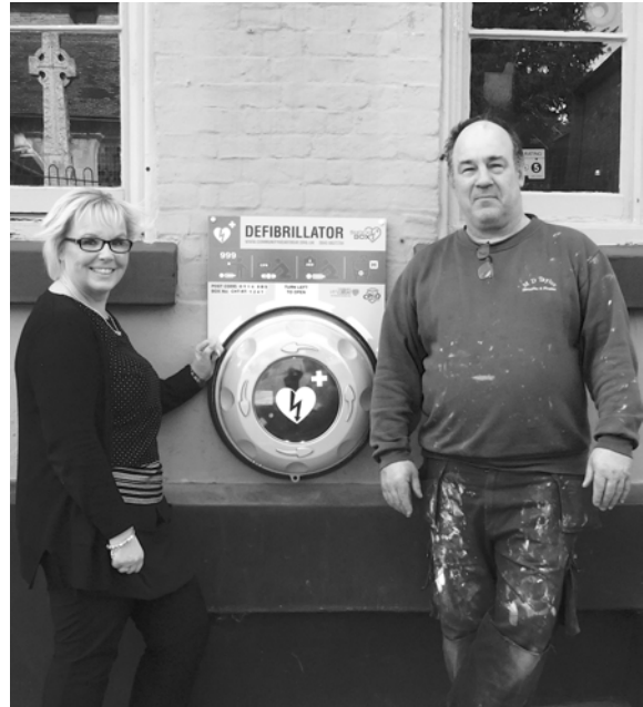
Wendy Satterley of The King's Arms and electrician David Taylor, who carried out the installation.
